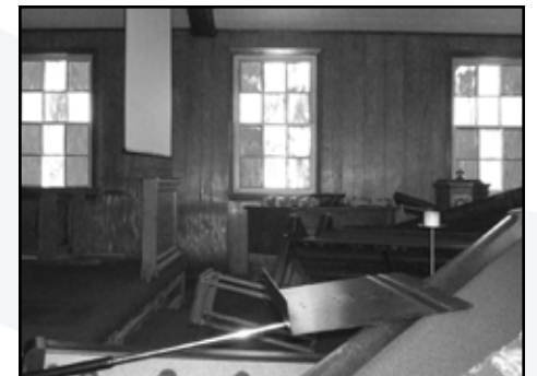
High water damaged most of the interior.
